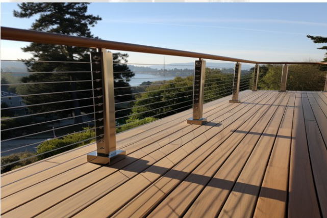
安全防护栏 Safety fence
