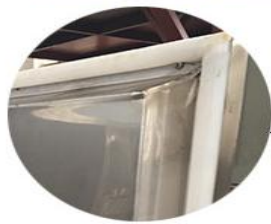
Door seam seal
