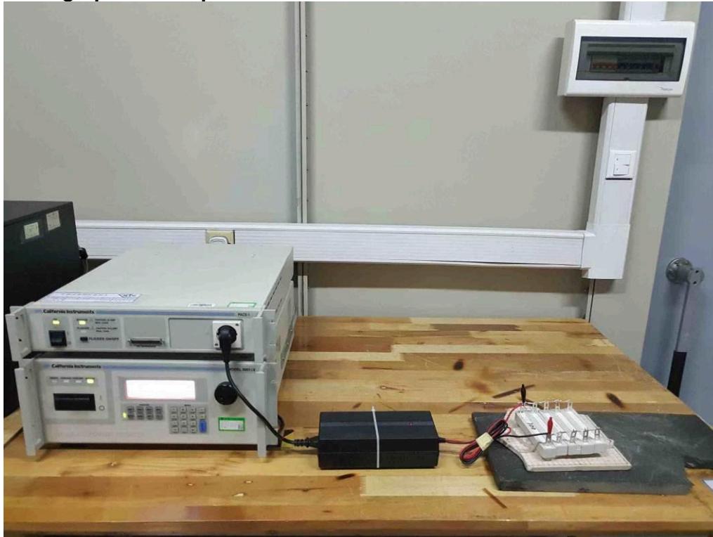
Photograph 8: Set-up for Harmonic on AC Mains
