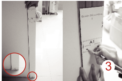
Put Scale Direction L on the desired location, make sure to suck the bottom line of A2 to the floor and mark the screw holes of A1 & A2 on.
