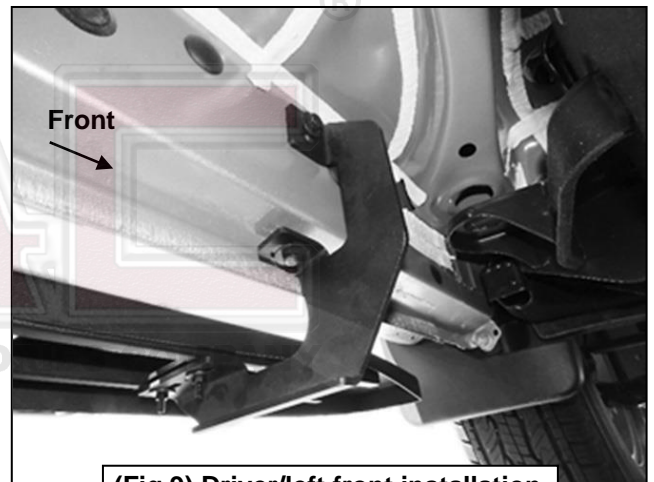
(Fig 9) Driver/left front installation
